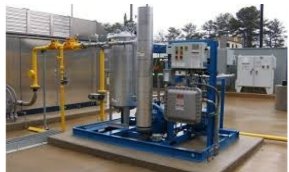
CNG – Natural Gas Compressor Dryer
