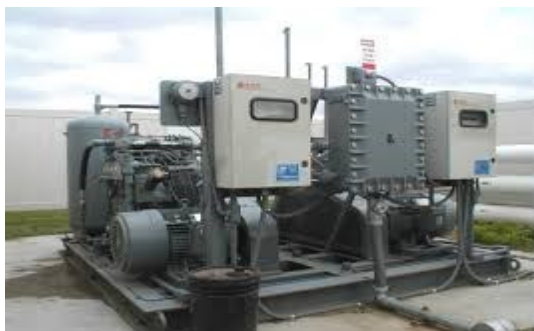
CNG – Natural Gas Compressor Unit
